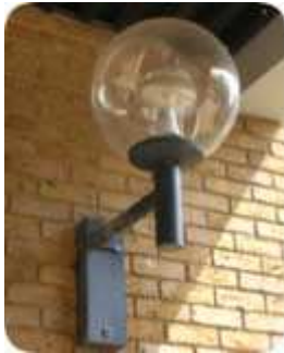
Local detail - Wall light fittings
